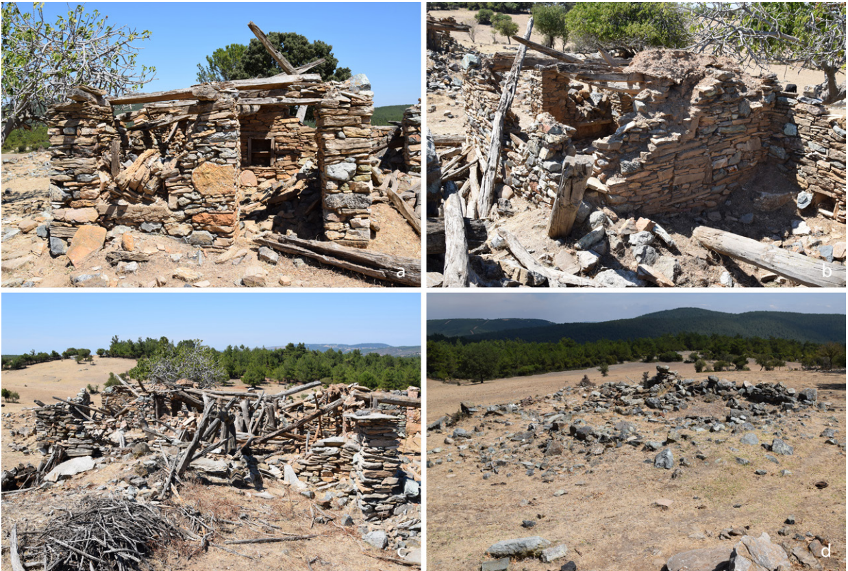
Figure 8. (a) Northwestern façade of the residential areas of building 1B (18 August 2016); (b) view of the residential areas of building 1B from the east (18 August 2016); (c) collapsed storage and utility rooms of building 1B, viewed from the south (18 August 2016); (d) collapsed condition of building 1E on 19 August 2016, viewed from the southwest.
