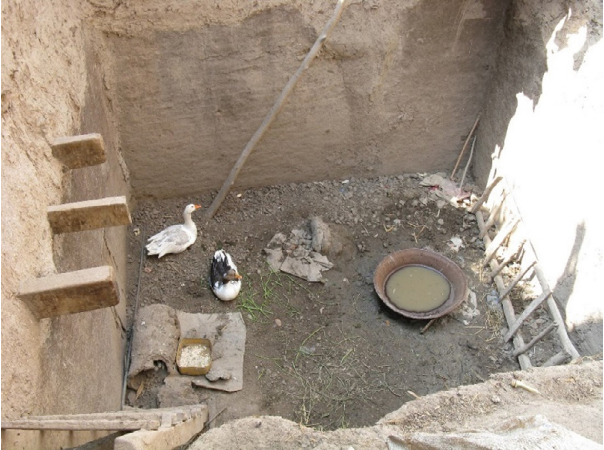
Figure 7. A collapsed first floor has created a courtyard where now animals are kept (Kom el Naggar, Lower Egypt). Photograph by the author.
