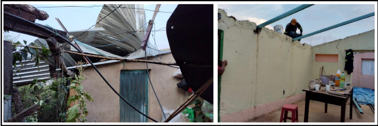
Figure 3. Galvanised sheet metal roof ruined by strong winds in Mazatlán Villa de Flores, Oaxaca (Photograph of the Project AZ 14/BE/23 Gerda Henkel Foundation).
