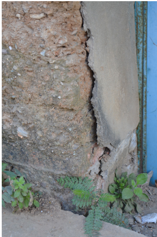
Figure 8. Cement plaster detached from the wall, creating a crack.
