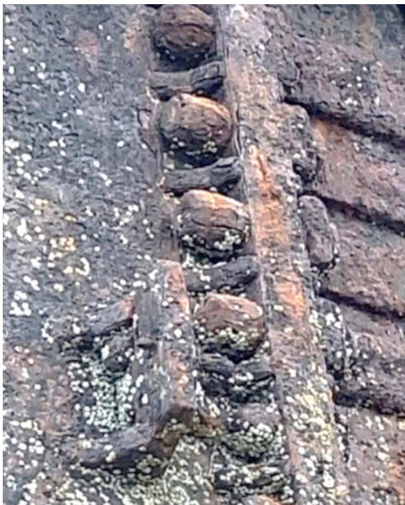
Figure 4.6: Corrosion of wrought-iron bolts. Copyright: Bella Romain.
