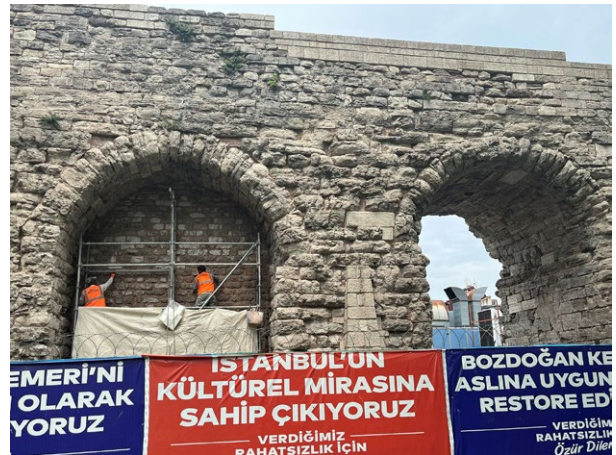
Figure 18. Restoration of the Valens Aqueduct (Bozdoğan Kemer), founded in 373 CE, situation in 2022 (photo. Mariëtte Verhoeven).
