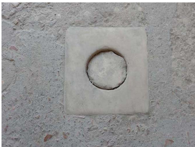
Figure 11. Pompeii, Domus Sirico (VII 1, 47), detail of inspection hole with marble cover (photo by the author, published with permission of the Ministero della Cultura - Parco Archeologico di Pompei).
