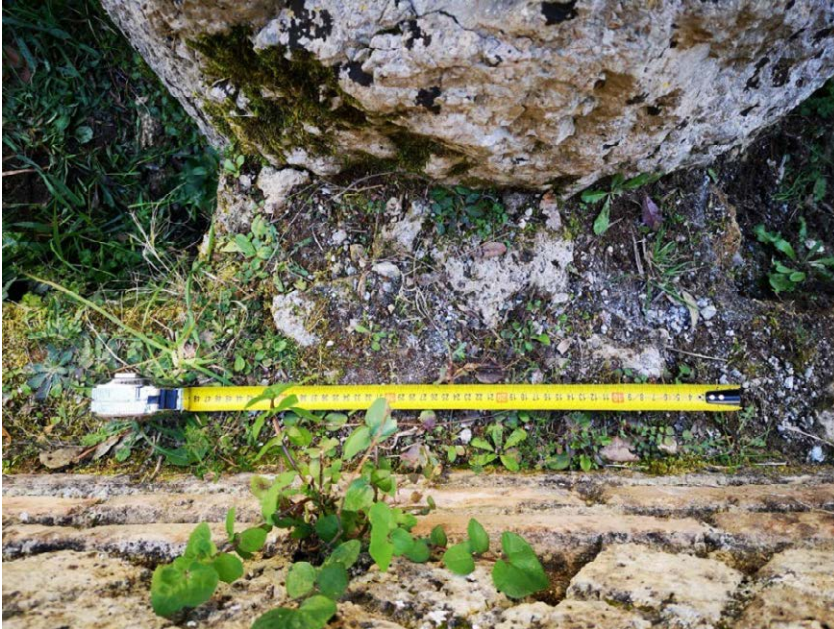
Figure 9. The sluce gate in mortar and calcareous tufa blocks which closes basin aVW to the west (photo by the author).
