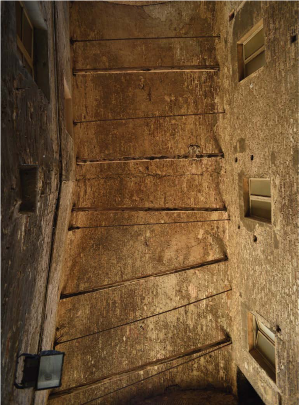
Figure 4.7 - Example of a wooden beam set inside wall masonry (Photo: Andrea Arrighetti)
