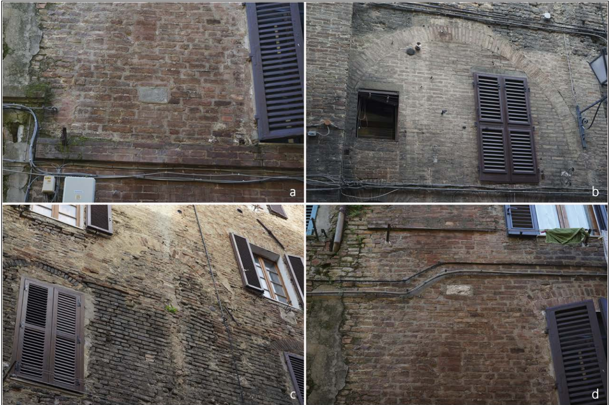
Figure 3.1 - Some examples of post-seismic techniques documented during the archaeoseismological fieldwork survey: bond stones (a and d) and relieving arch (b and c).
