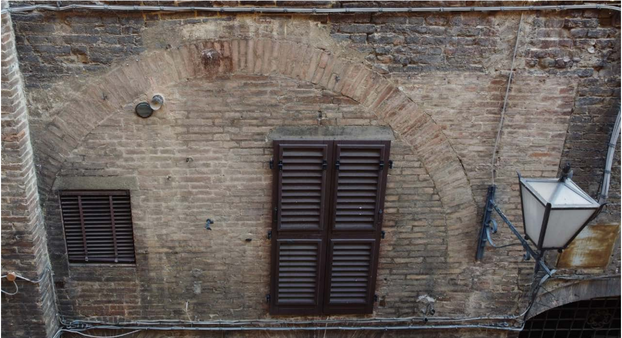
Figure 4.9 - Relieving arch inserted into the façade of a building in Via Pendola (Photo: Gianluca Fenili).
