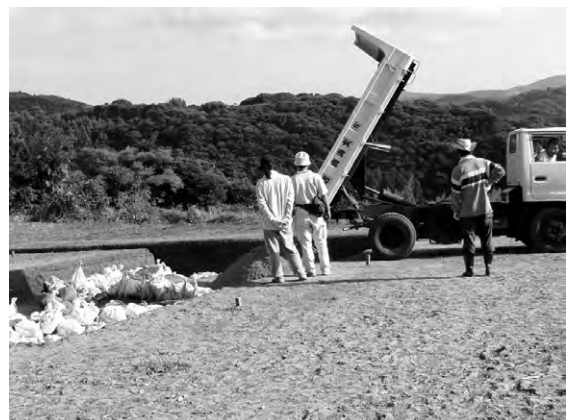
Figure 9.16 26th September: Laying out sandbags and sand; the excavation squares were then backfilled until the next year's investigations
