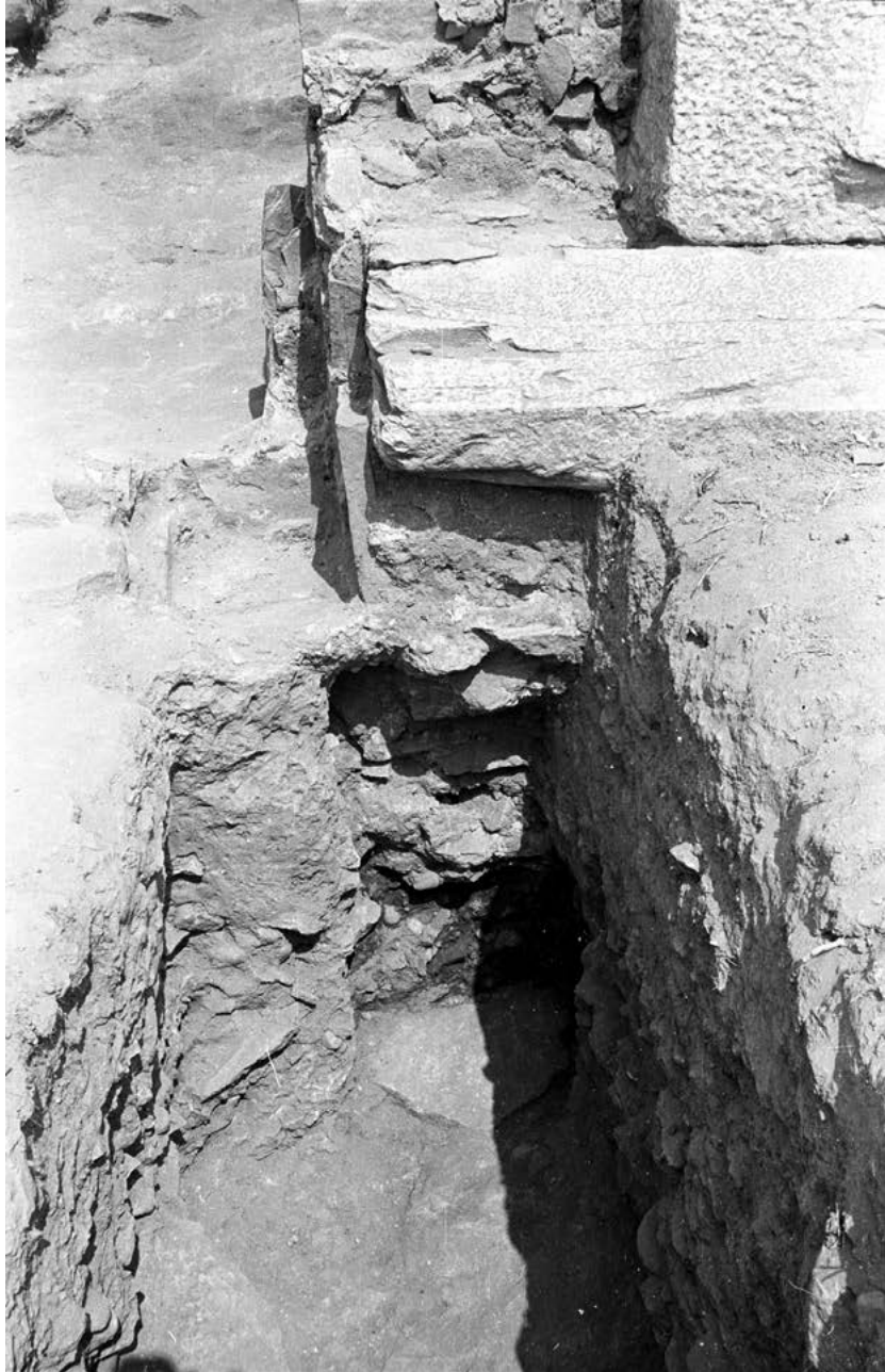
Figure 18. Door to center room behind podium, Phase III door jamb built into podium base course with deposits below.
