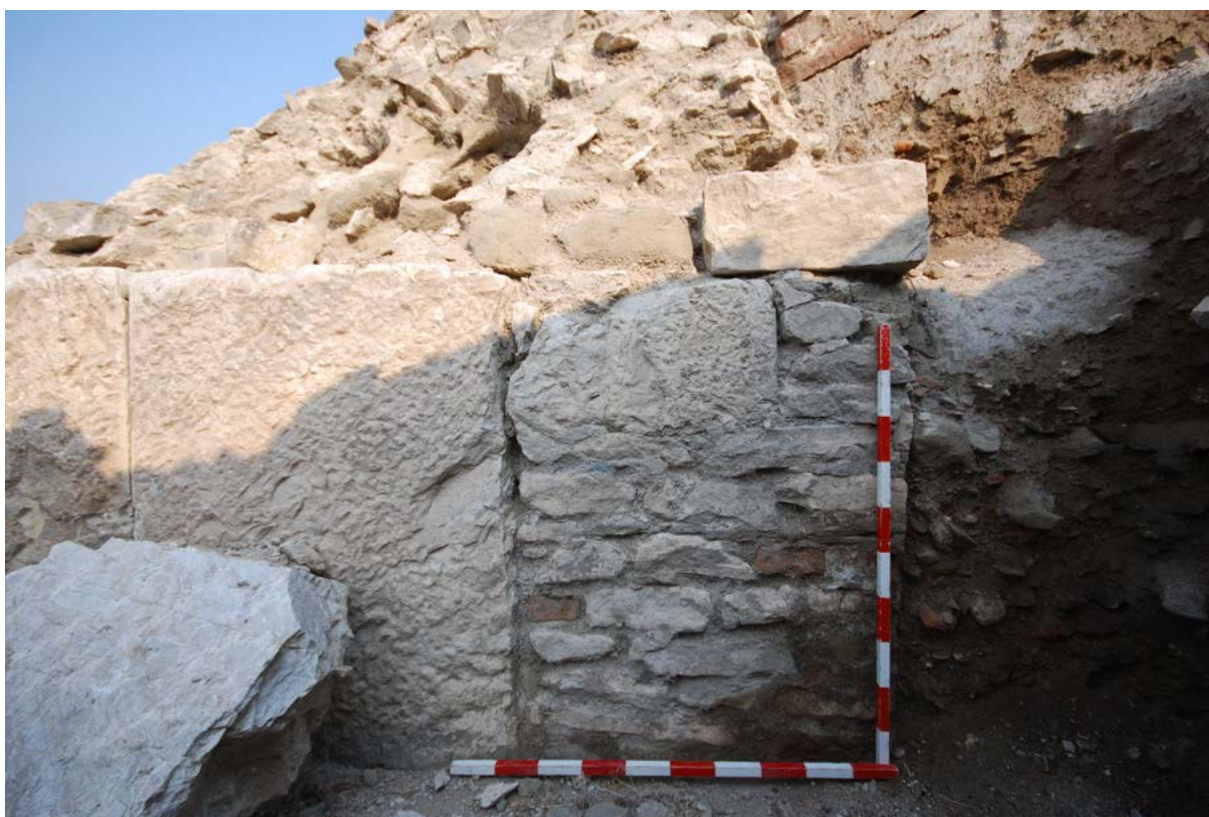
Figure 67. North side, east corridor, added masonry at end of vault. Stair at left.
