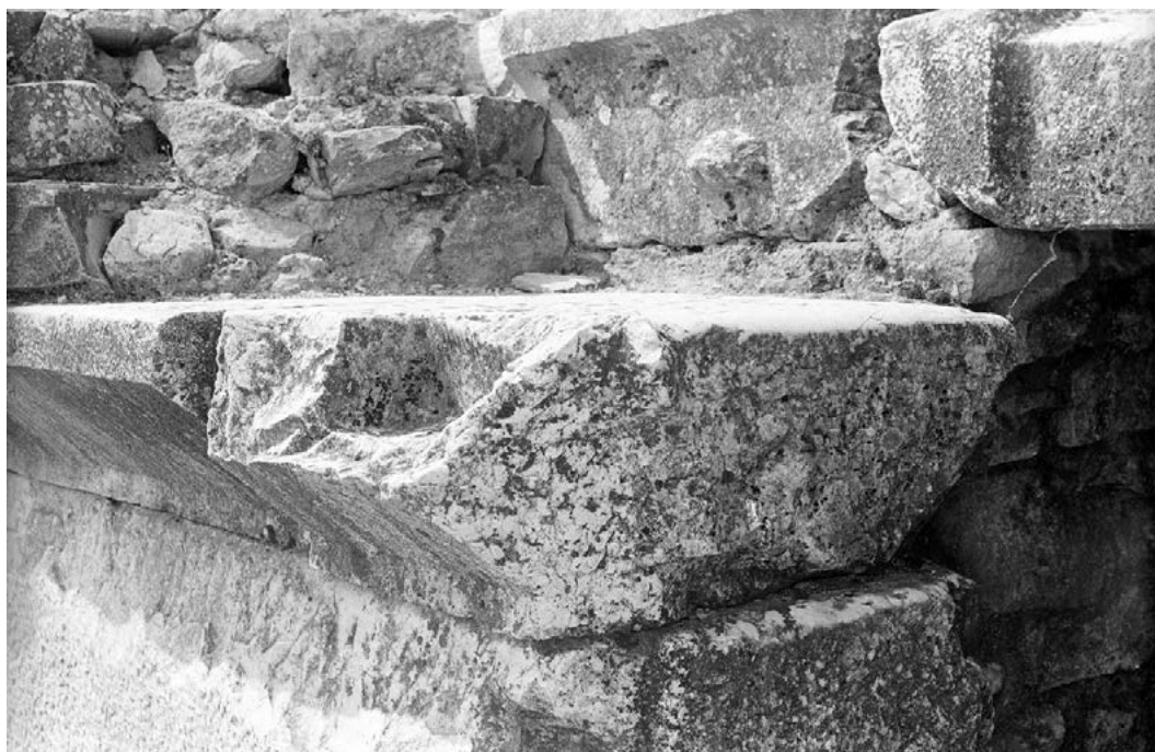
Figure 252. Crown course of podium broken, at west refuge.
