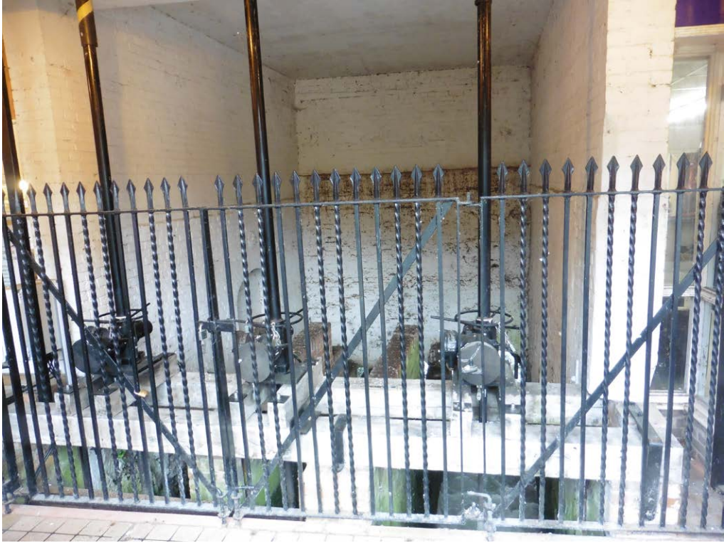
Figure 13.16: Sluices for hydro-electric power turbine at Bishop's Mill (© The Author)
