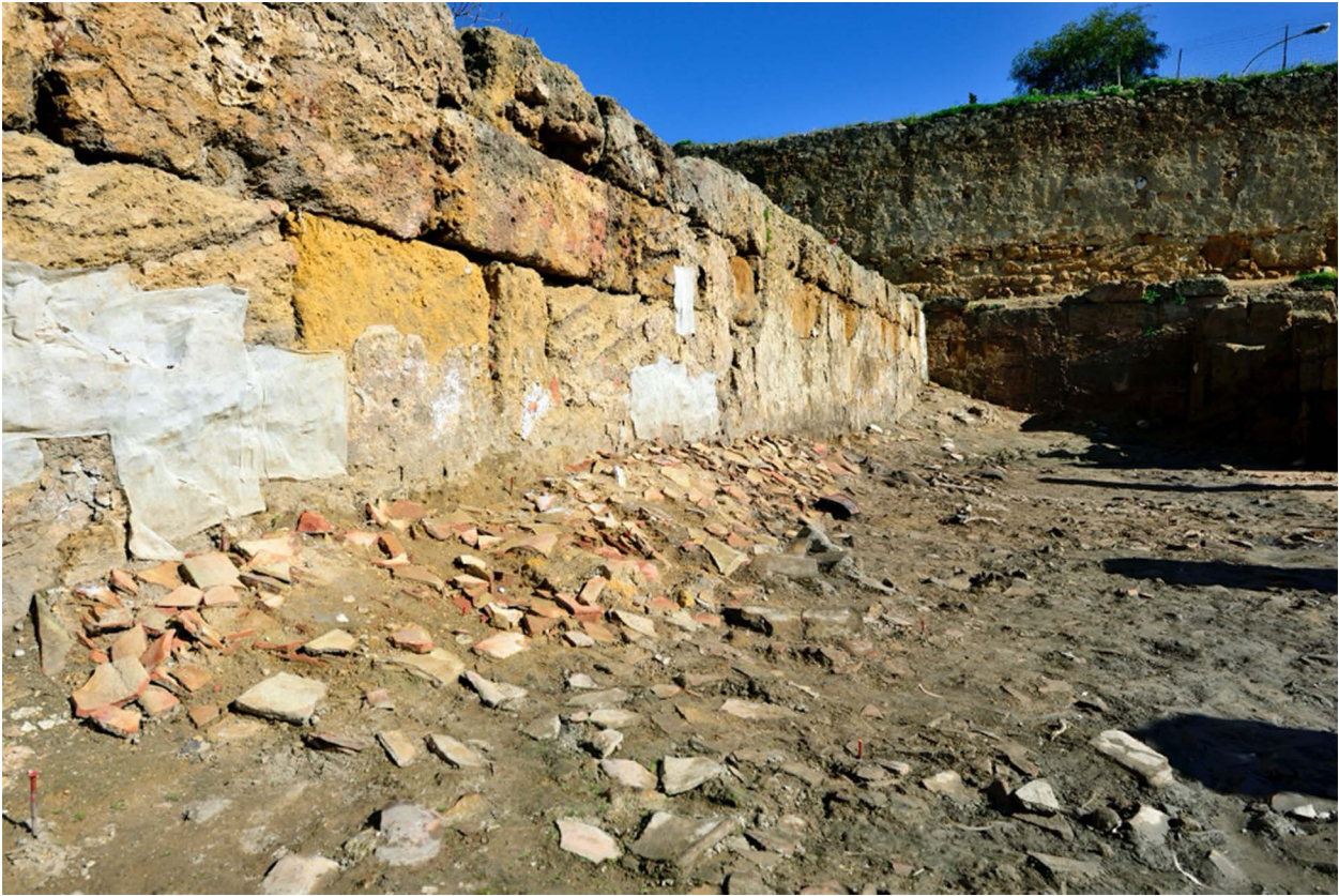
Figure 5 – Hellenistic-Roman sanctuary in Agrigento: the fallen roof of the northern portico
