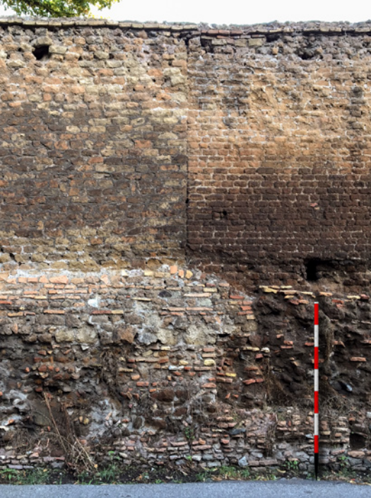
Figure 3. South-east frontage (PR2) - detail: connection between the walls in small blocks (right) and the earlier structure in roughly refined rubble (left).
