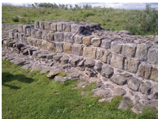
88. Different stages in building of the Wall: broad foundation, narrow foundation and narrow wall
