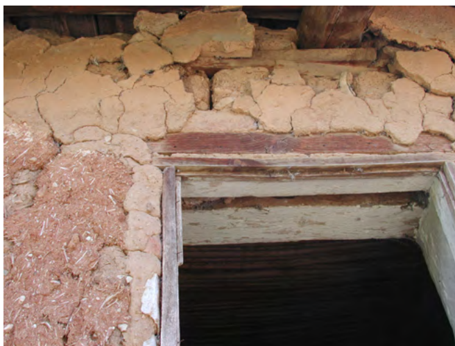
Figure 8. Cracks around an opening in a traditional house (Kovačevo, Bulgaria) (photo by S. Prévost-Dermarkar).
