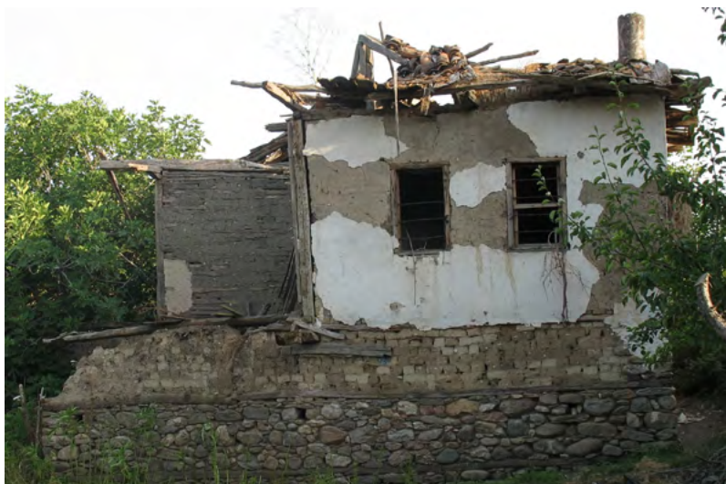
Figure 9. A traditional house with a stone foundation (Kovačevo, Bulgaria) (photo by S. Prévost-Dermarkar).
