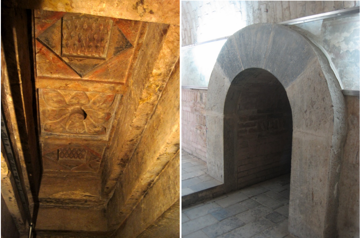
Figure 2-15c (left), stepped roof of the Yi'nan tomb. Photograph by the author. Figure 2-15e (right), barrel vault of the Xingyuan tomb. Photograph by the author.
