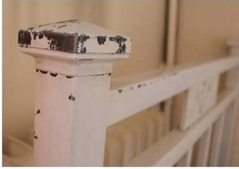
Fig. 7. Oil Paint loss and Scratches
