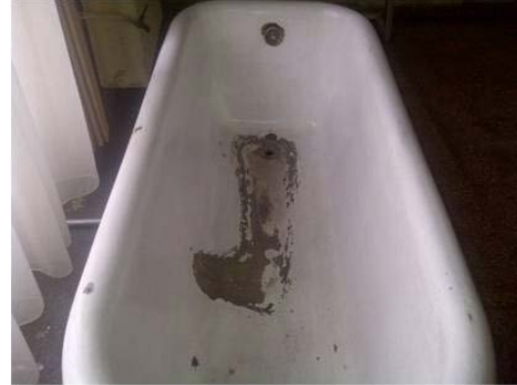
Fig. 8. Dirt and Stains from Corrosion
