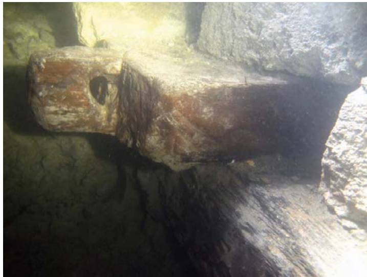
FIG. 23. WOODEN BEAM WITH THE CROSSPIECE IN THE BASE OF THE SOUTH-EASTERN WALL OF TOWER 1
