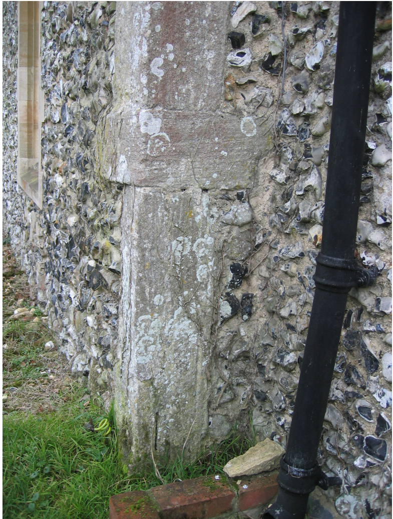
Figure 1.10. Detail of the lowest three stones (in the long and short Anglo-Saxon style) in the south-west nave quoin at Stretthall church (TL 484 398) in Essex (after Potter, 2009c). From the lowest stone upwards, the bedding orientations are BVFR, BH, BVFL. The rock type used is Barnack Stone, imported into the region.
